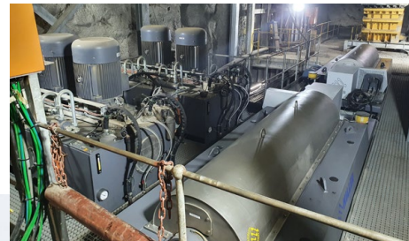
HILLER decanters in 1,600 metres underground
