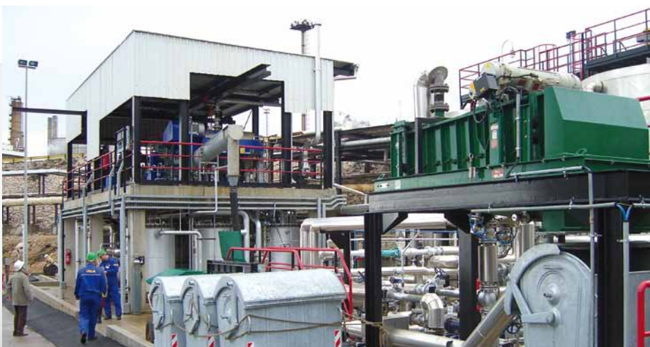
Explosion-proof oil sludge treatment plant in a refinery
