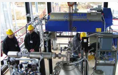
Explosion-proof oil sludge treatment plant
